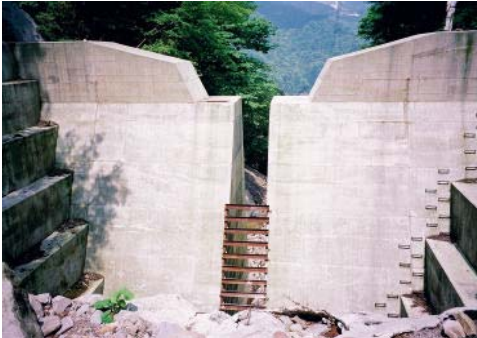
Figure 4.7. Concrete slit-type sabo dam. Steel bars were installed at the slit after debris flow was found to pass through the slit (Photo 5; Mizuyama [No 1], 2008).
