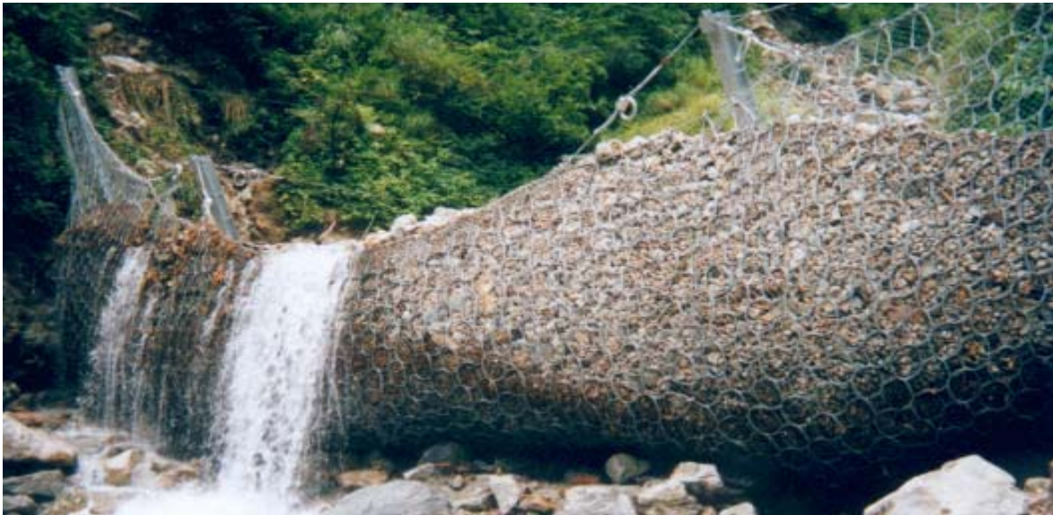
Figure 4.12. Example of flexible ring-net barrier after debris-flow event. Approximately 980 cubic yards of material is retained by barrier in photo (Figure 1; Roth et al., 2004).
